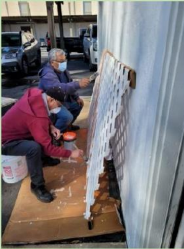
[Above] Another task as a result of the windstorm back in January. Lloyd & Kenny are shown painting a fence replacement from the yard of the church parsonage.
