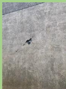
Hole on gym wall
